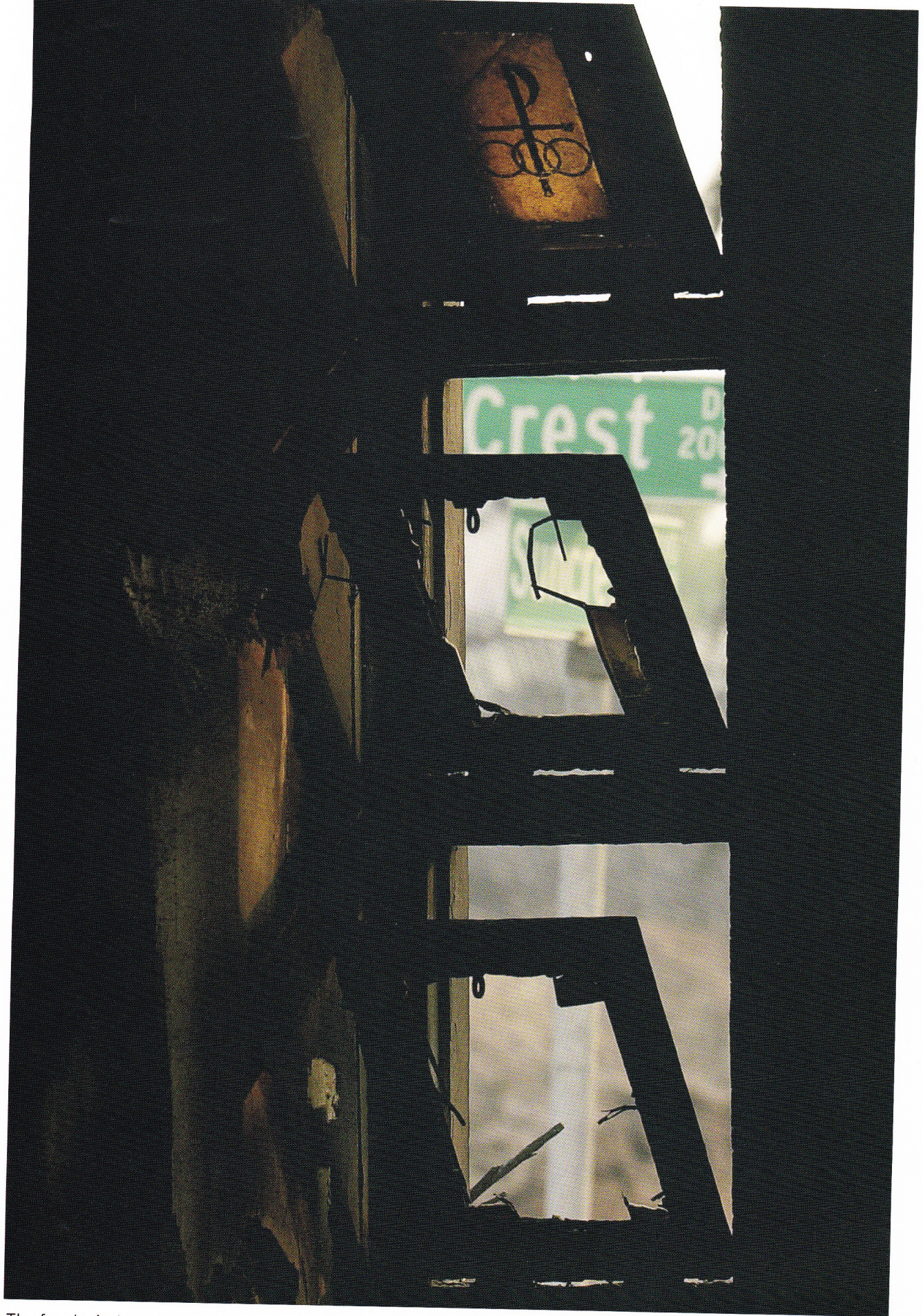
The front windows were blown out of the St. Louise de Marillac Roman Catholic Church in Crest, where the sanctuary and rectory were heavily damaged. PHOTO BY PEGGY PEATTIE
