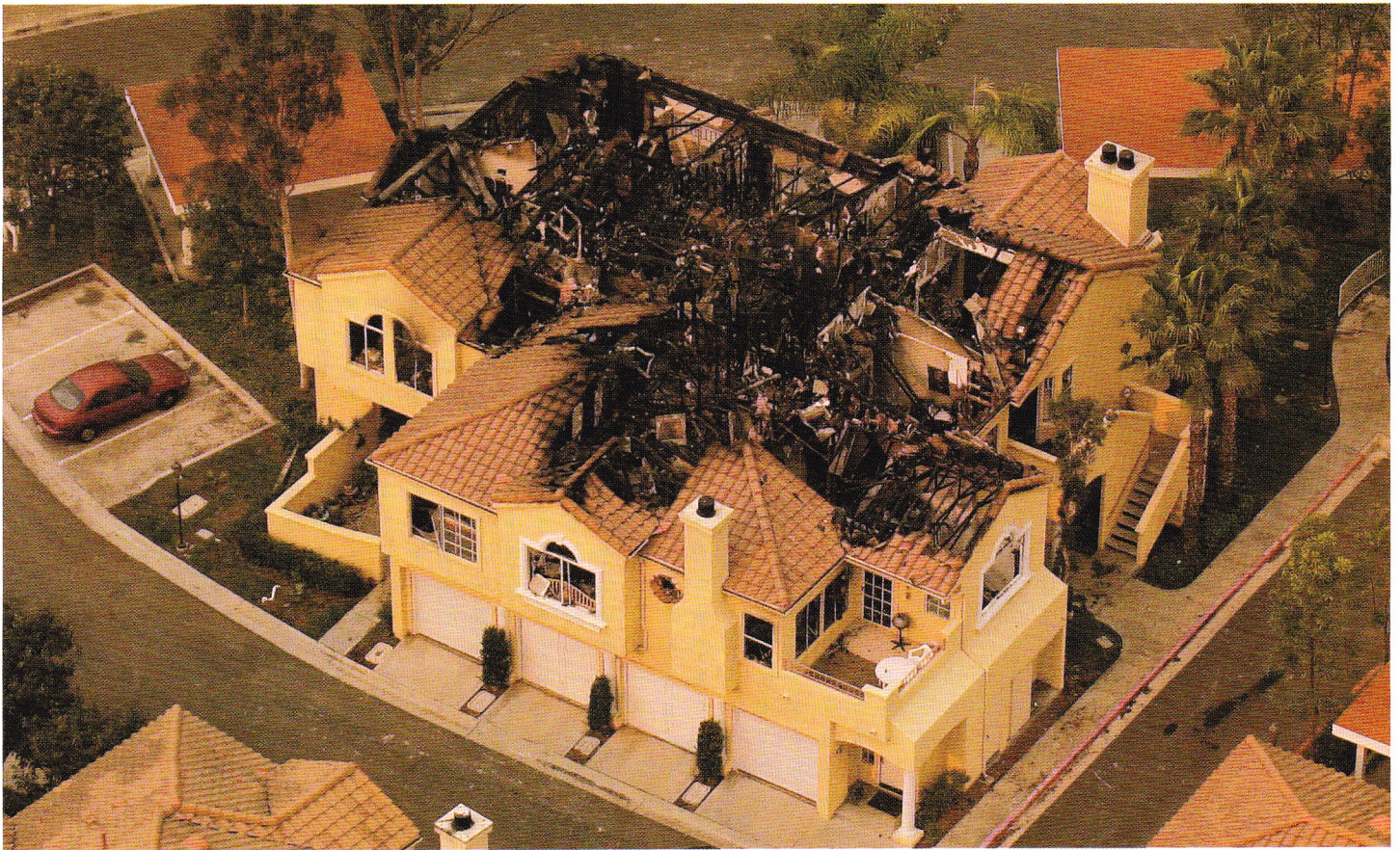
A residential complex in Tierrasanta, near the intersection of Portobelo Drive and Camino Playa Cancun, was heavily damaged. PHOTO BY JOHN GIBBINS
