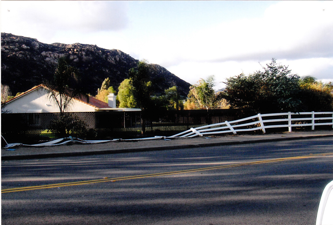
South Grade Road by Deer Creek Melted Plastic Fencing
